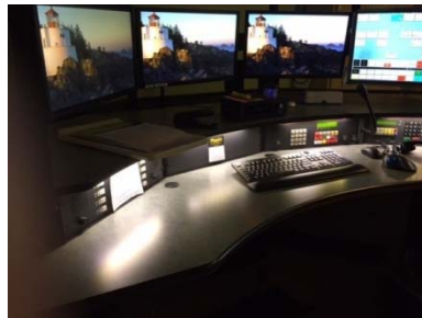
Indirect LED lighting in riser shelf with dimming
